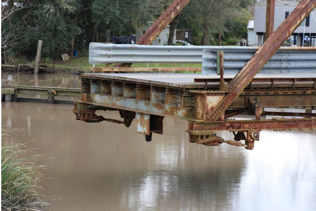
Condition Photo 10: End of the main truss span showing paint failure as well as the condition of the live load bearings and locks.
