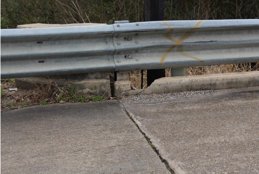
Condition Photo 16: Spalled concrete curb and debris north approach at the joint for the approach slab and bridge approach spans.
