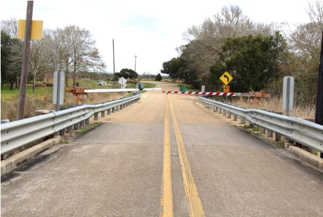
Condition Photo 1: North approach span looking north. Note metal guardrail, approach slab, and traffic gates.
