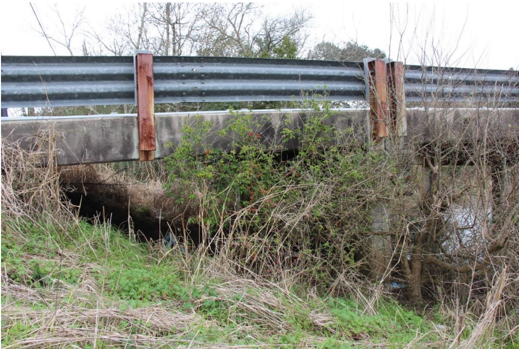
Condition Photo 17: Vegetation growth at the north approach bents; similar condition at south approach bents.
