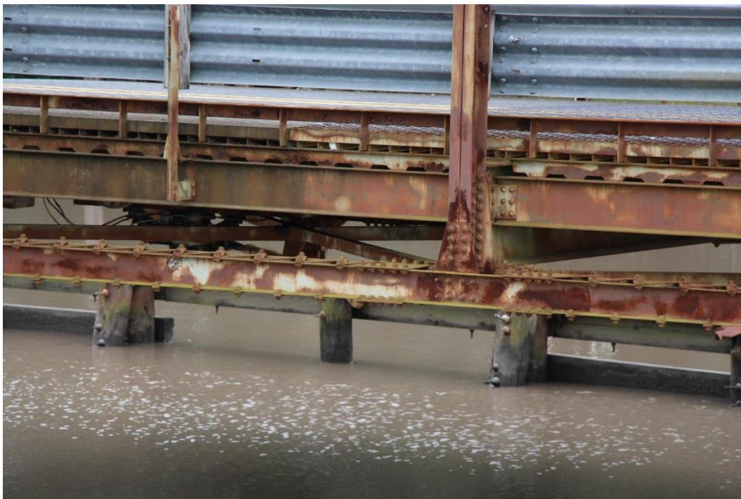
Condition Photo 9: Lower chord paint failure of the main truss span.
