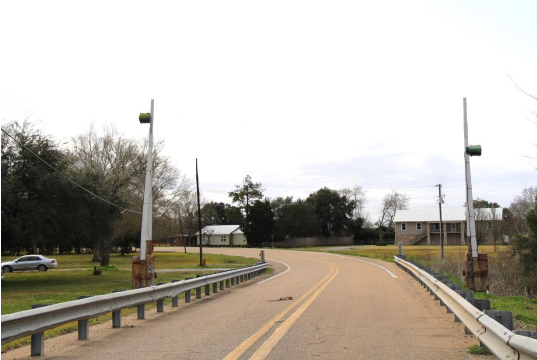
Condition Photo 2: South approach roadway looking south; note guardrail and traffic gates.
