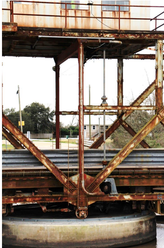
Character-defining Feature Photo 3: Design and construction of a through truss swing span. Detail showing the track system and shafts and couplings that connect operating machinery in the operator's house to machinery and gears supported on the pivot pier.
