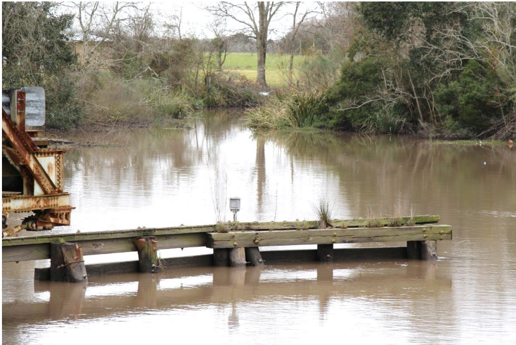
Condition Photo 23: Timber fender system vegetation growth.
