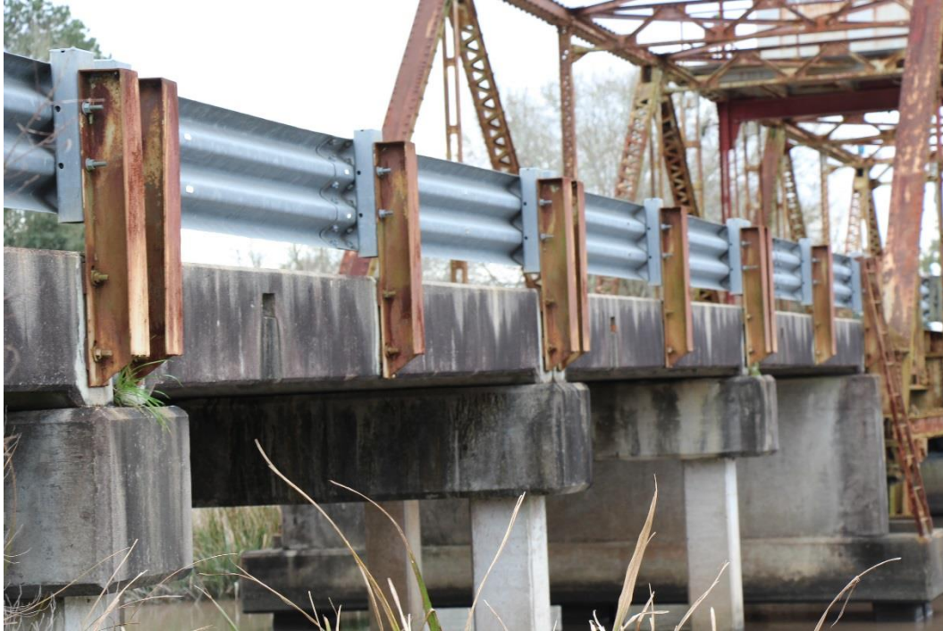
Condition Photo 18: Water staining and vegetation growth on approach Bents 3-5 and Pier 1
