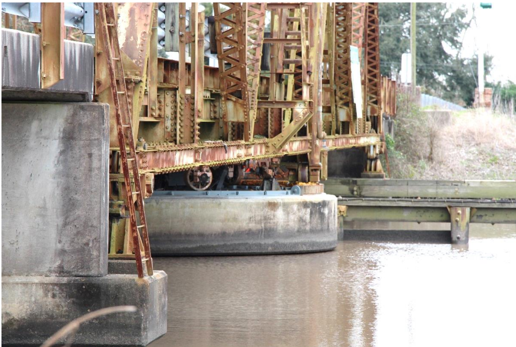
Condition Photo 25: Swing and approach span piers and condition of the swing span.
