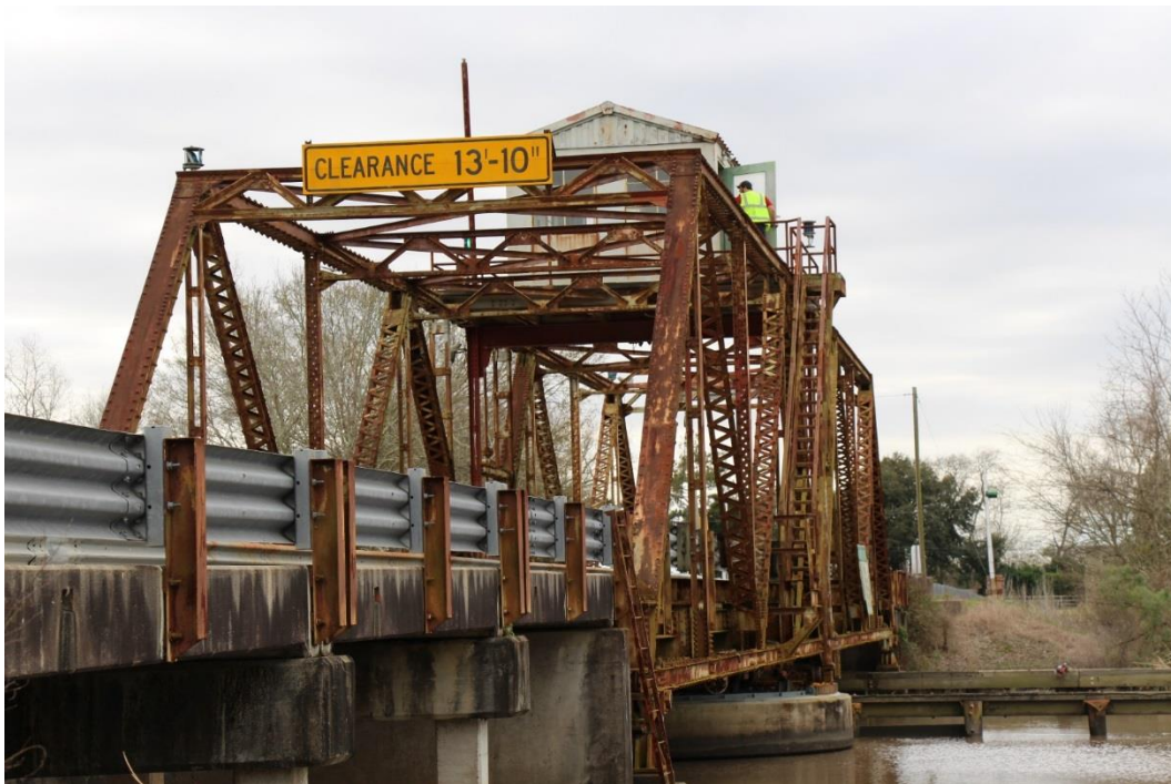
Condition Photo 5: Elevation view of the north concrete approach spans and main span truss, exhibiting concrete staining and paint failure.
