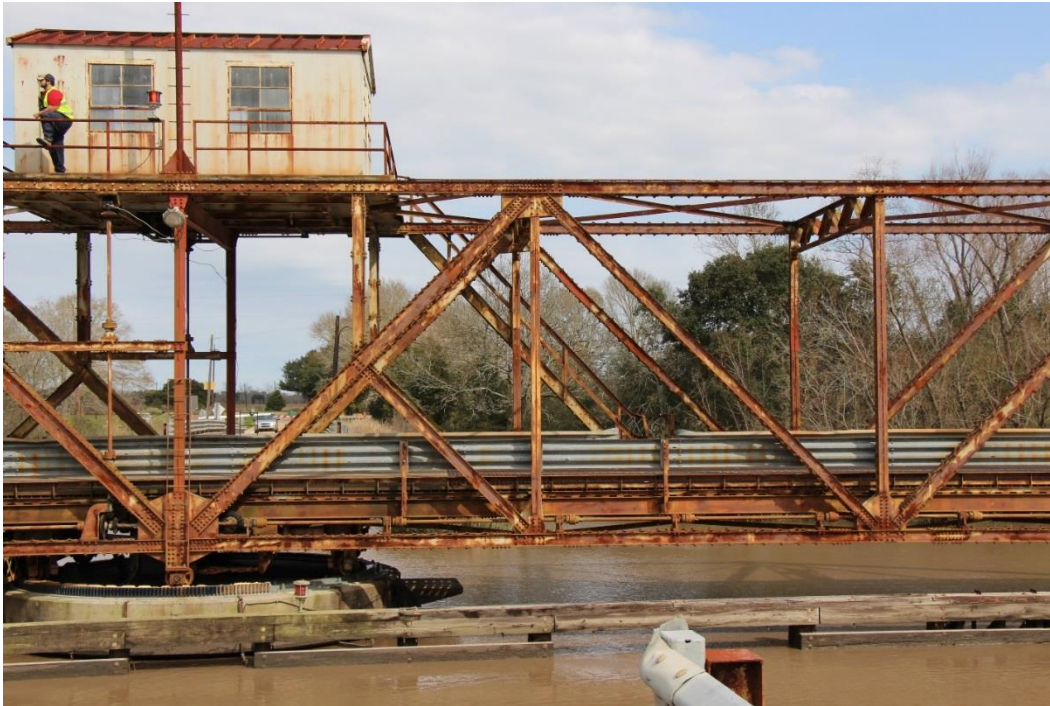
Character-defining Feature Photo 2: Design and construction of a through truss swing span. The main swing span (shown in open position) featuring rim-bearing turning mechanism with a pivot pier. This roller-and-track system guides the motion of the bridge when it opens and closes. Shafts extend from the operator's house to the turning mechanism.
