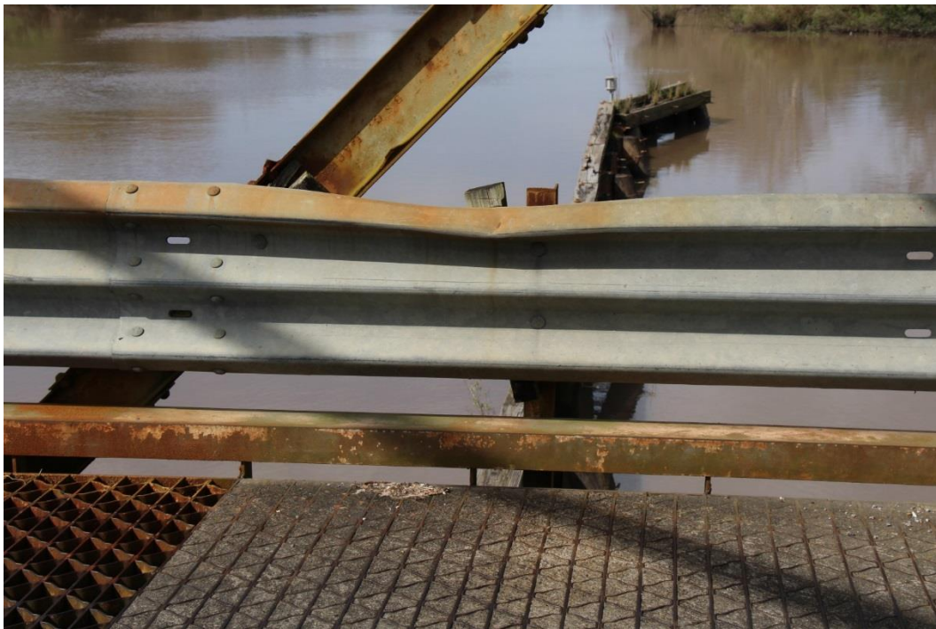
Condition Photo 13: Damaged guardrail on the main span.
