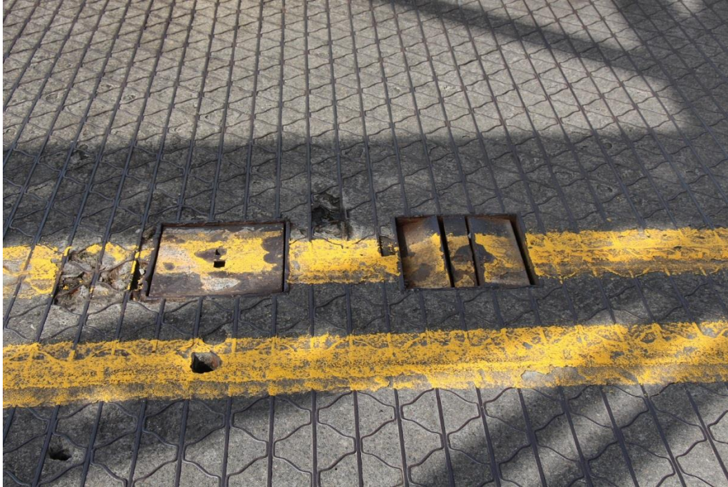
Condition Photo 14: Concrete filled metal grid deck wear and spalling on truss span.
