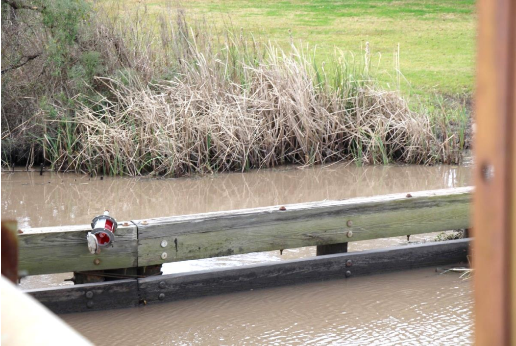
Condition Photo 24: Broken navigation light on the timber fender system.
