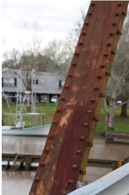
Condition Photo 8: Diagonal member of the main span truss paint failure.
