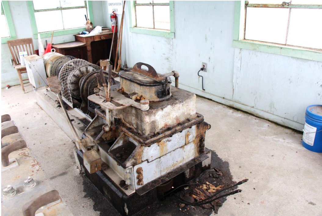
Condition Photo 22: Motor and machinery in the operator's house.
