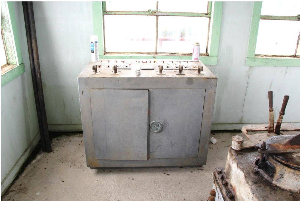
Condition Photo 21: Control console in the operator's house.
