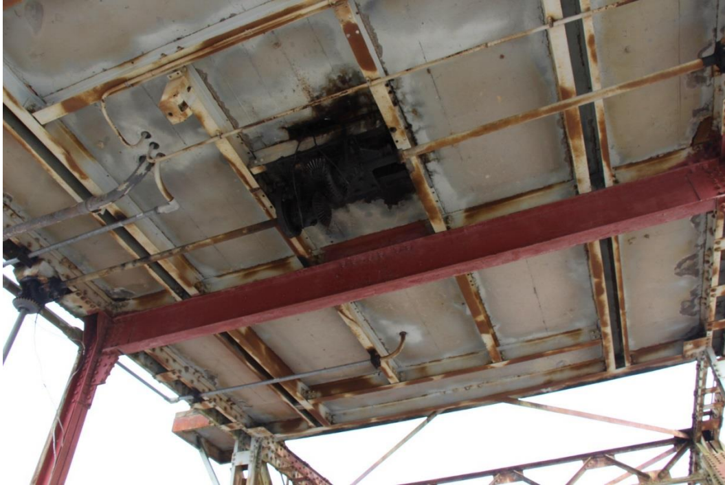
Condition Photo 20: Gears and shafts for the swing span under the operator house at the center on top of the truss; note the newer steel beam and column which replaced in-kind deteriorated original steel members.
