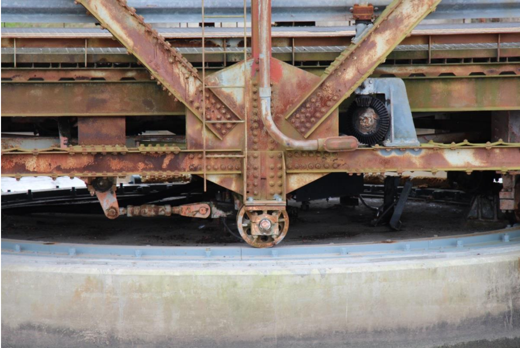
Condition Photo 6: Close-up of the rollers and steel ring track at the center pivot pier (Pier 2) under the truss span.
