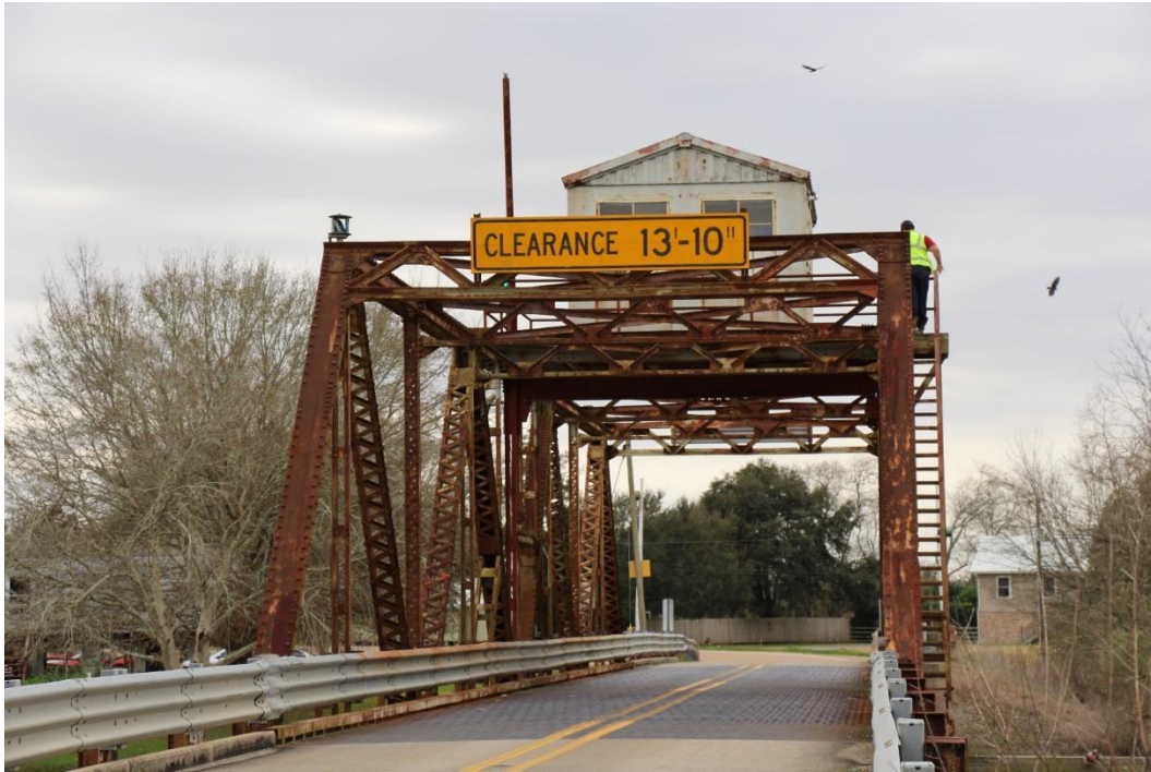
Condition Photo 4: Main span truss paint failure.
