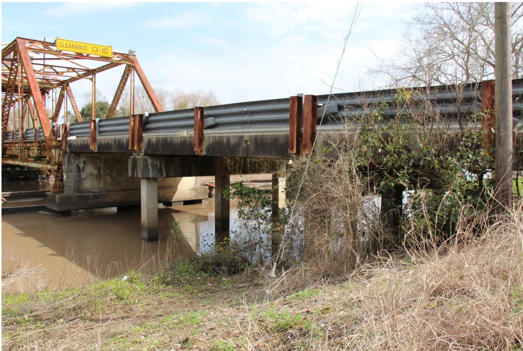
Historic Fabric Photo 4: Concrete substructure and concrete slab approach spans. This photo also shows the added guardrail, which is not historic fabric.
